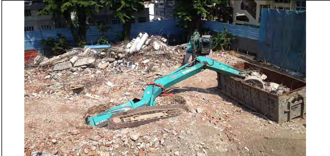
A building was being demolished using an excavator standing on the first floor. The floor collapsed bringing down the building. The excavator fell into the basement and was partially buried by rubble, trapping the operator in the cab. Unfortunately by the time rescuers reached the operator he had died.
